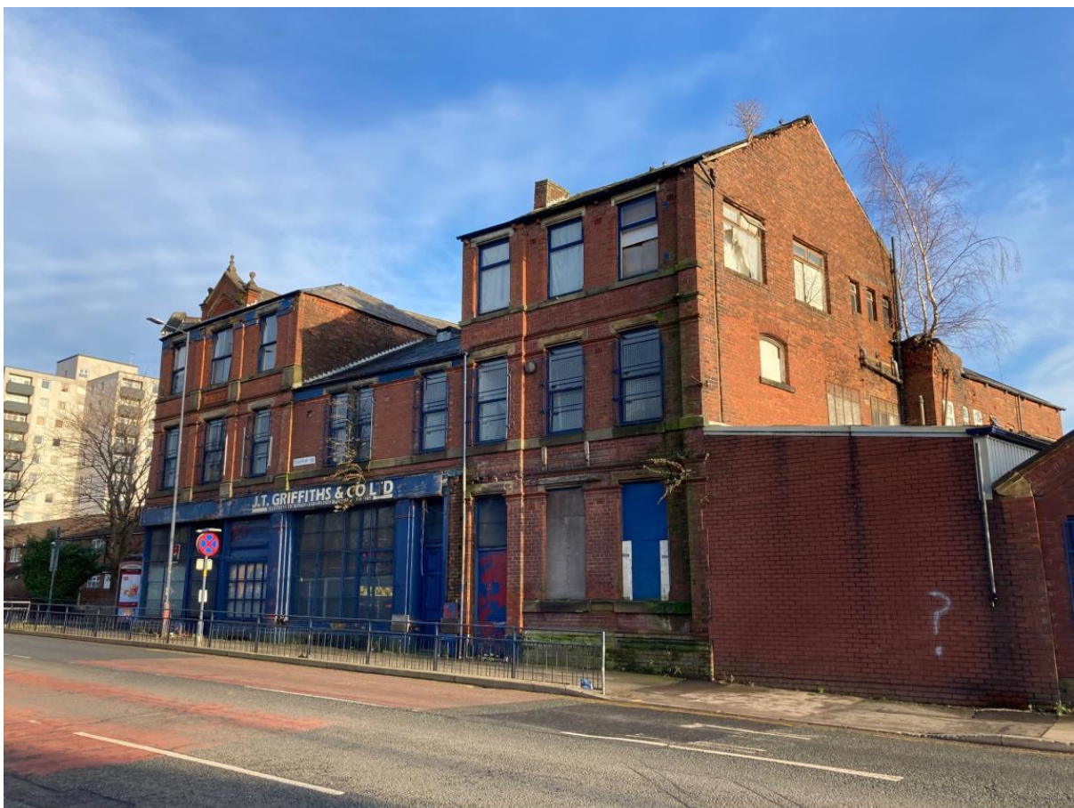
Photo 2: View of the front elevation of the building viewed from Stockport Road
